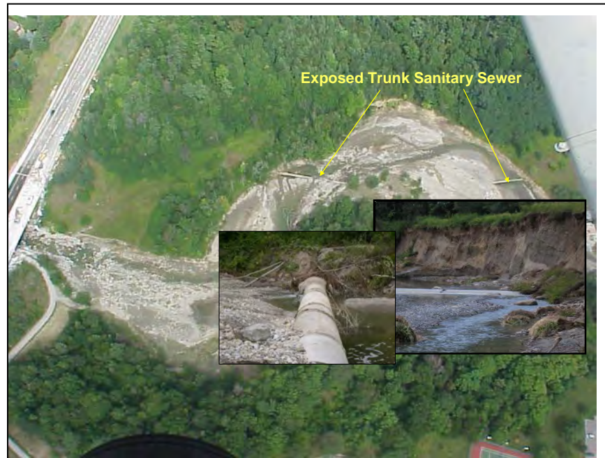
Figure E5-8: Picture and Location of STS erosion in Highland Creek watershed caused by Aug 19 th , 2005 storm extreme weather event
