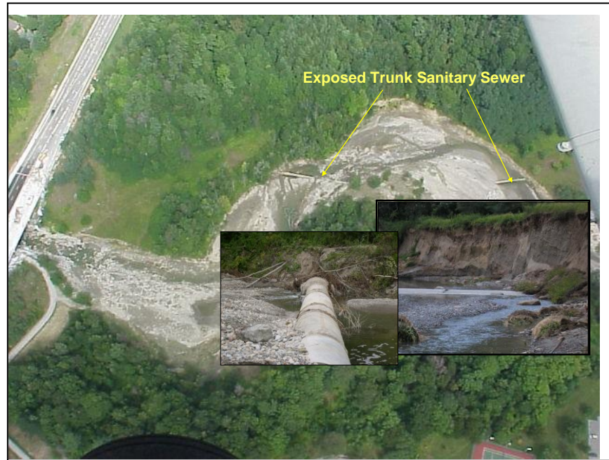
Figure E2.9: Picture and Location of STS Erosion in Highland Creek watershed caused by Aug 19th, 2005 Storm Extreme Weather Event
